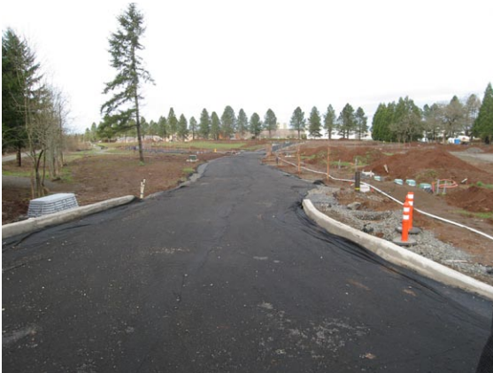
Figure X. The photo above was taken during the construction phase at Pringle Creek when pervious streets were covered with filter fabric to avoid excess soil filling the voids in the pavement.
