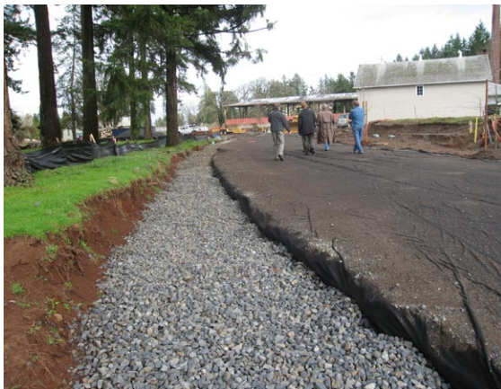
Figure X. The pervious paving used at the Pringle Creek Sustainable Community in Salem, Oregon uses crushed basalt aggregates as a structural base which also acts as water storage.
