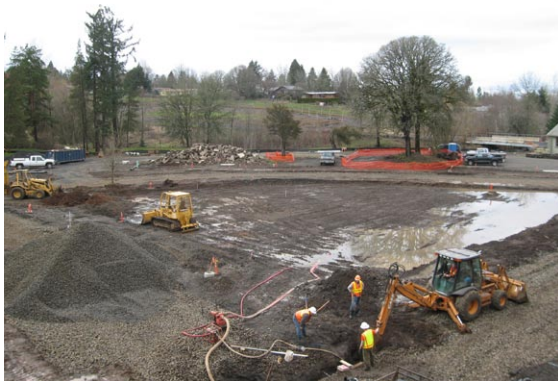
Figure X. The standing water seen here is actually the high water table revealed during the winter. The finished road surface is only a few inches above this point yet stays dry as water travels through the street section and surrounding soils via interflow, emerging in the banks of pringle creek almost visible in the distance beside the trees. The surface of the creek is only a foot or two lower than the water table, but sufficient to draw down the water if interflow is not impeded.
